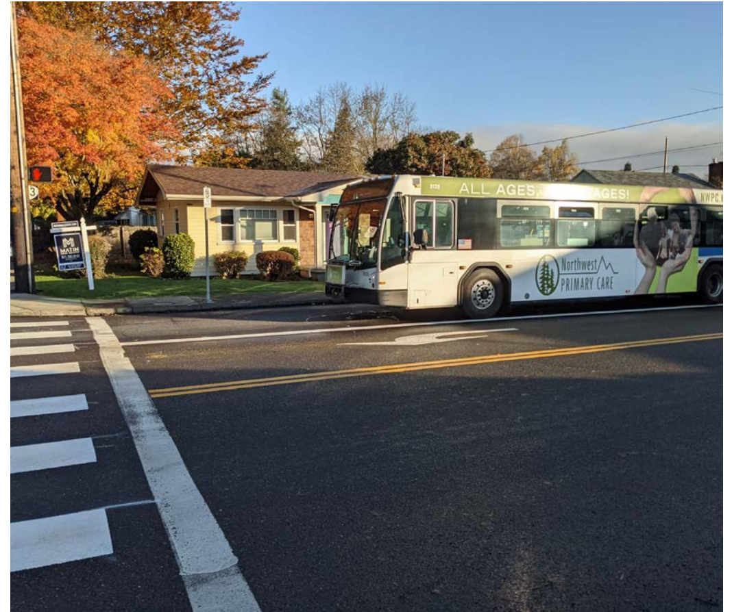
Restriping to provide a left turn pocket at NE Prescott St & NE 82nd Ave
